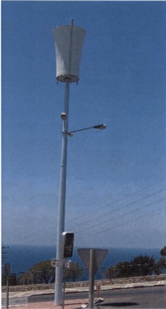
Exhibit 8. The antenna is wider than, and out-of-scale to the pole. This design is prohibited.
